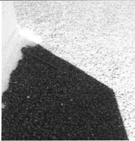
Flashing seal cracking
